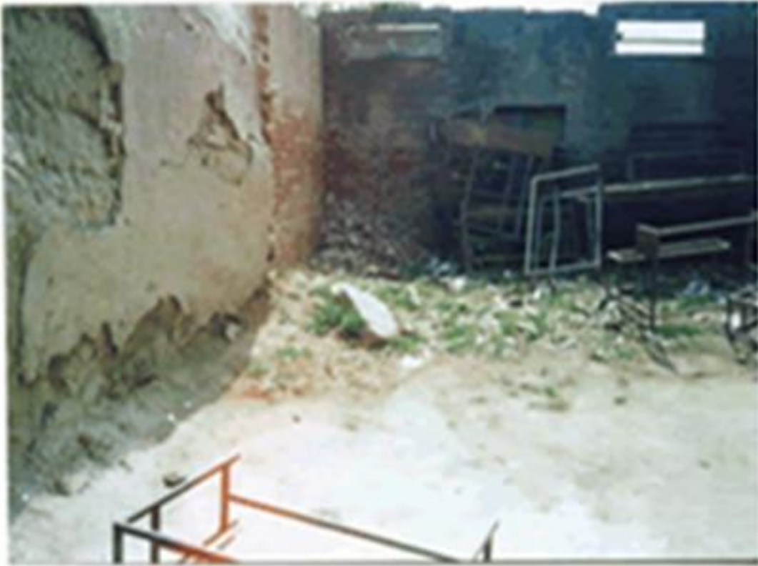
Before starting the project (1999) the school was in desperate need of repair and maintenance
